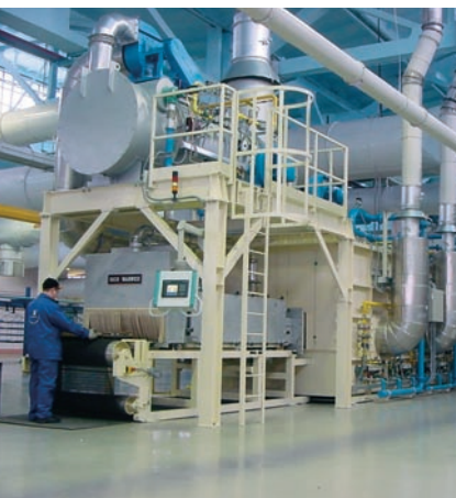
A continuous-belt furnace is used for high-volume production of brazed copper-brass heat exchanger cores. (Photograph courtesy of SHAAZ.)
